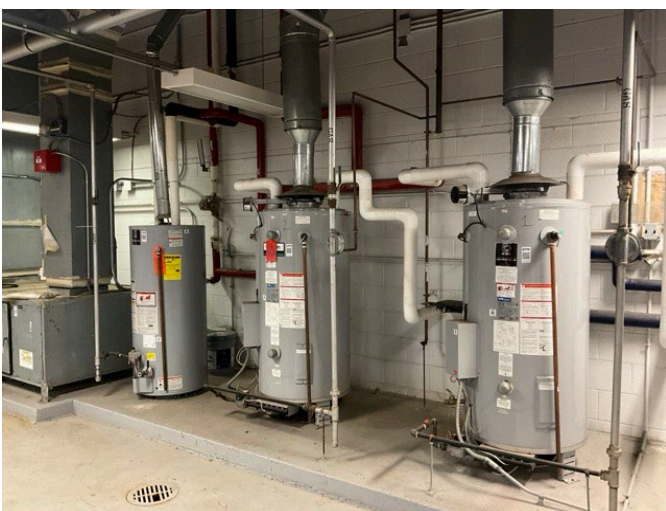
29 - DOMESTIC WATER BOILERS
