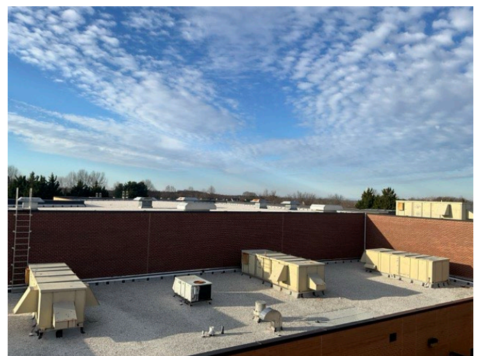
30 - ROOFTOP MECHANICAL EQUIPMENT
