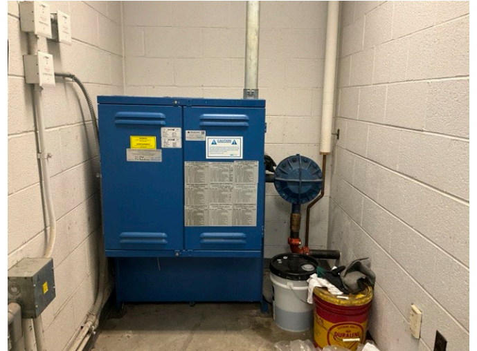
26 - ELEVATOR CONTROL ROOM
